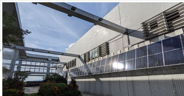
▲ In Hong Kong, we installed 40 solar panels on the rooftop of BEA Tower in Kwun Tong, which is capable of generating around 8,400 kWh in renewable energy annually.
